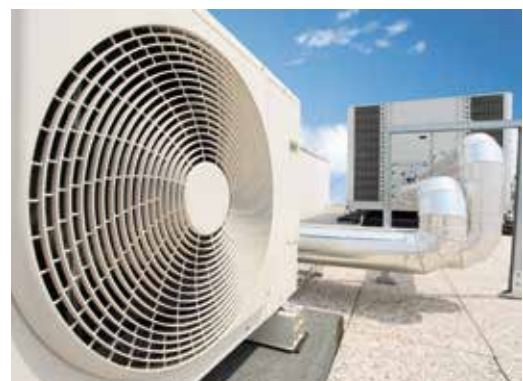
A/C units on a flat roof.
