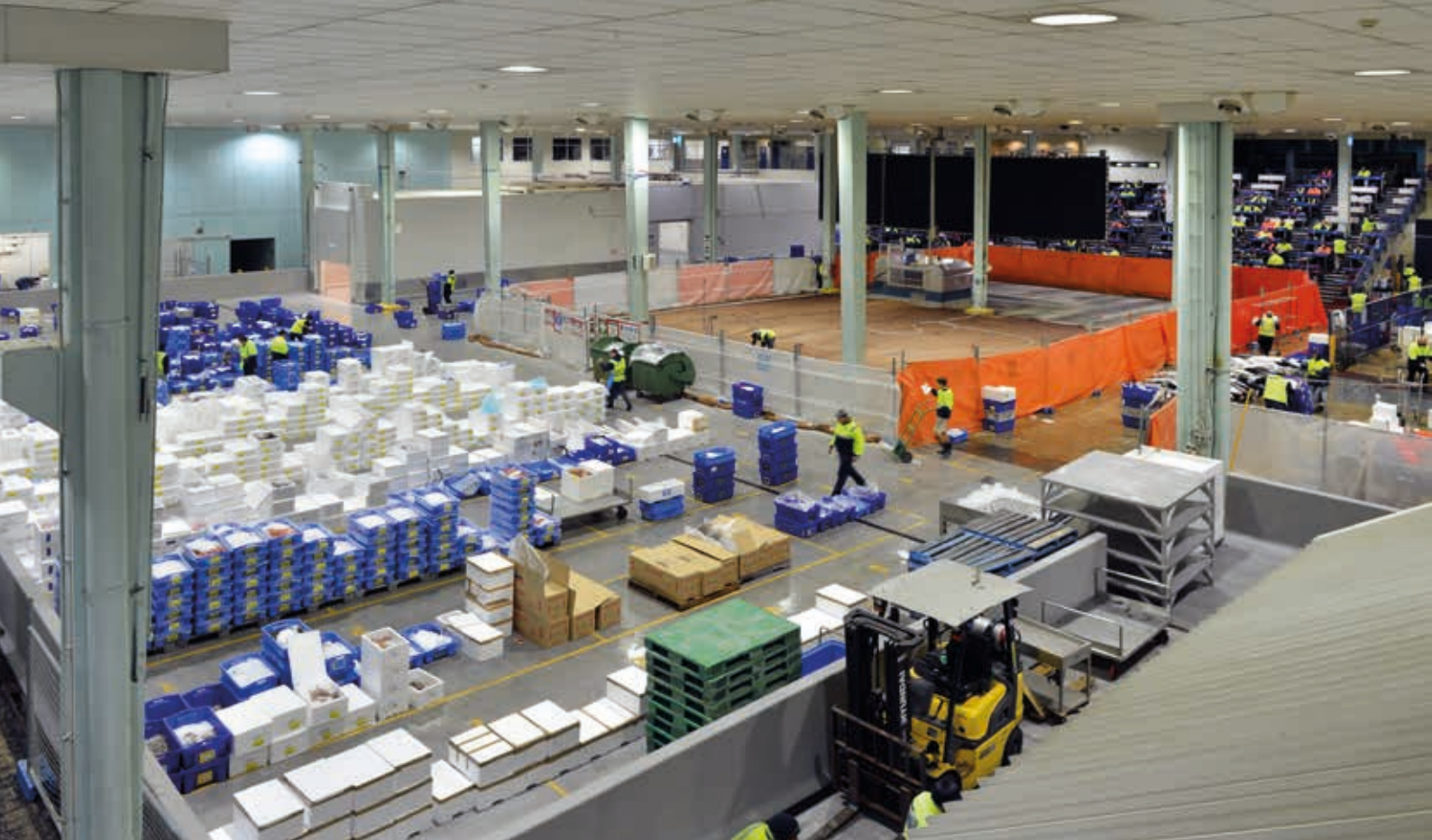
Operations continued during flooring works on a fish market floor refurbishment site
